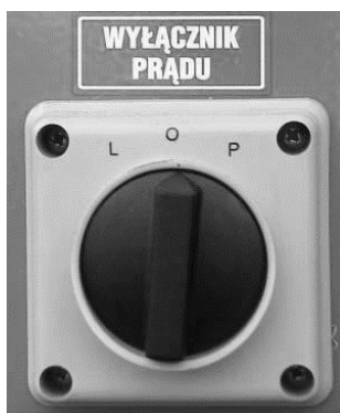
Figure 2 – current switcher before connecting the machine to the network
